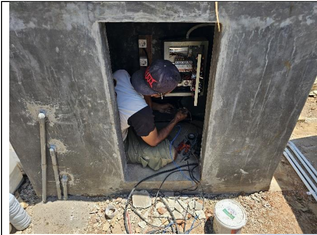
Setting Control Panel dan Pompa
