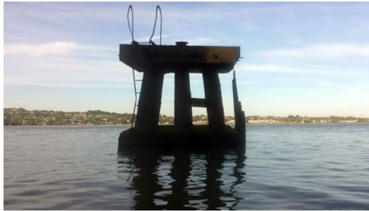
Gambar 1-2 Mooring Dolphin Sumber : Google image
