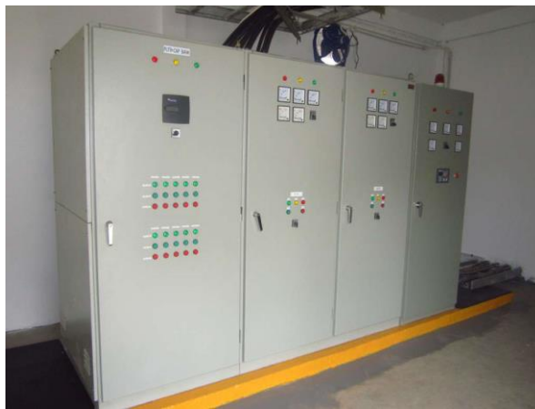
Gambar 2.7 Low Voltage Main Distribution Panel (LVMDP)
