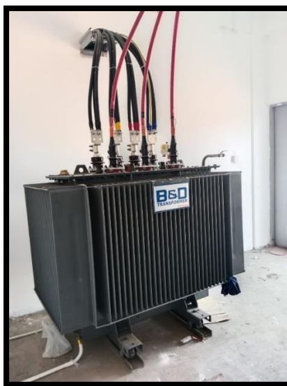
Gambar 2.4 Transformator Step Down Gedung
