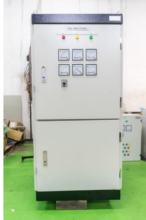
Gambar 2.8 Sub Distribution Panel (SDP)
