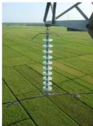
Gambar 3. 3 Isolator Kaca 150 kV
