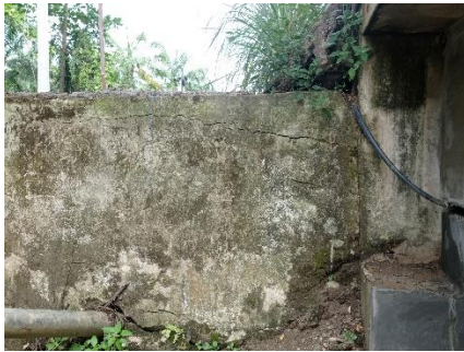
Dinding penahan tanah retak
