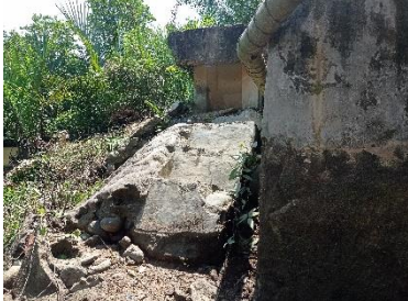
Dinding penahan tanah pecah
