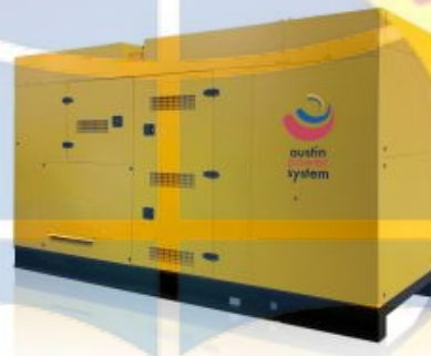
Gambar 2.6 GENSET RS Hermina Pasuruan
