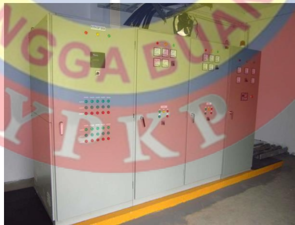
Gambar 2.7 Low Voltage Main Distribution Panel (LVMDP)
