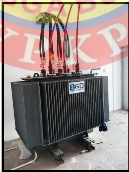
Gambar 2.4 Transformator Step Down Gedung
