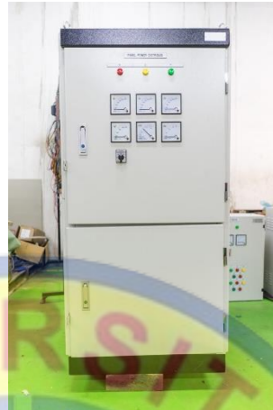
Gambar 2.8 Sub Distribution Panel (SDP)
